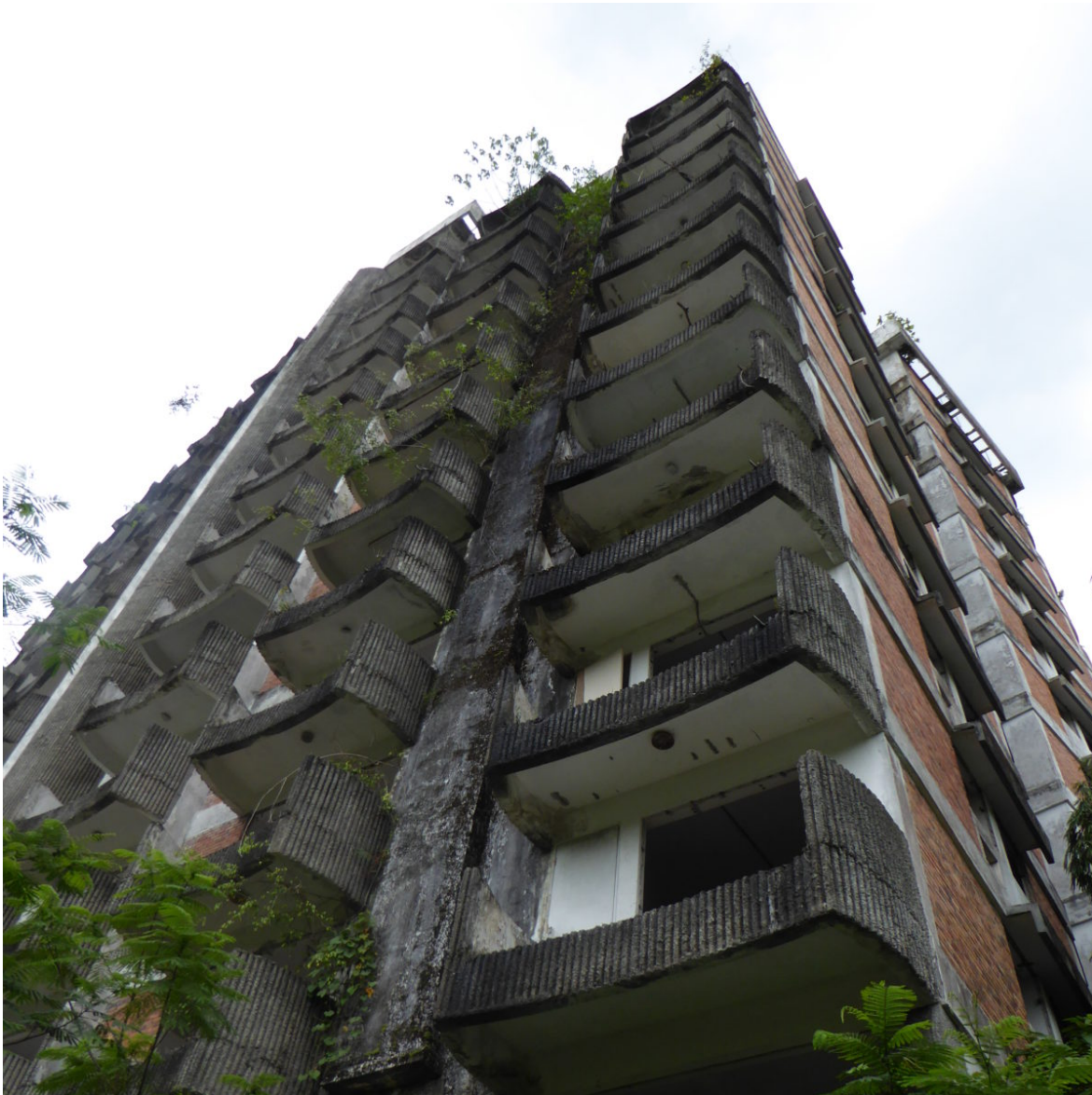
Highland Towers, Malaysia © Veronika Fendel
